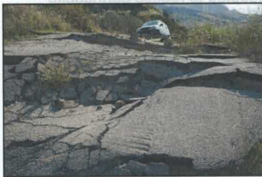
Damage after an earthquake
